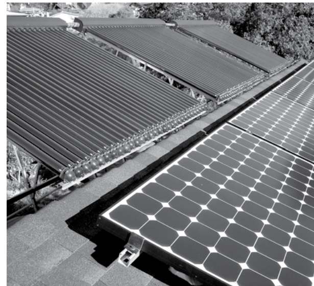
FIGURE 6-5. EVACUATED-TUBE COLLECTORS (ABOVE) AND PV ARRAY (BELOW)
